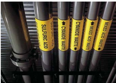
CPVC chemical process piping
