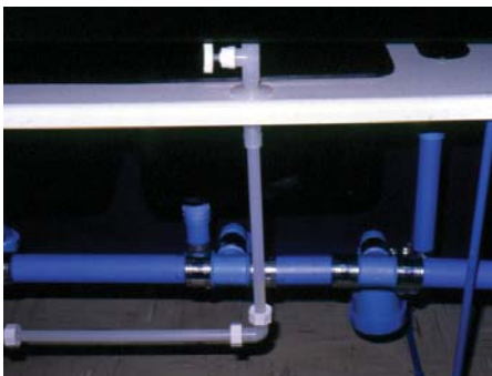
PP chemical waste and high purity piping under-bench lab systems
